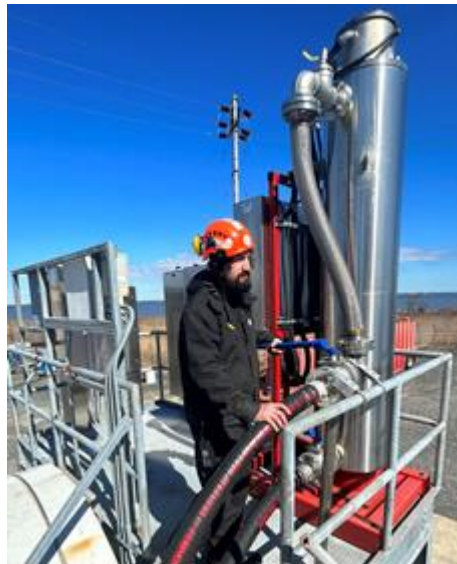
Figure 4 Vertical heater operation to aid in heat transfer during decanting
