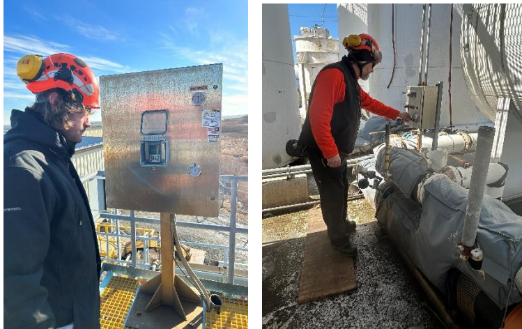
Figure 3 Flow rate and positive displacement pump operations between the test tank (left) and tank farm (right)
