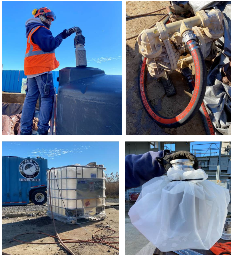
Figure 5 Secondary wastewater treatment phase of cement runoff with PAC in dilution tank
