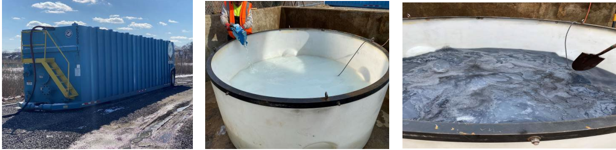
Figure 4 Primary wastewater treatment phase of cement runoff with PAC
