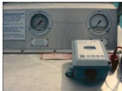
Flow meter mounted on control stand
