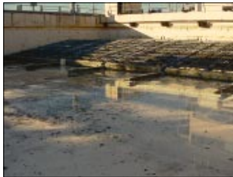
The empty test basin reveals the beaches awaiting repair.
