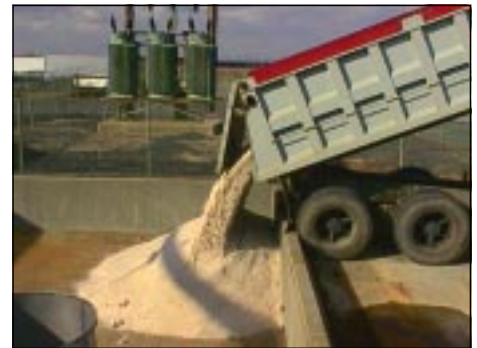
Please pass the salt! A load of salt arrives to raise the basin water salinity.
